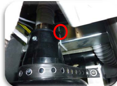
Picture 4: Open the distributor unit and unclamp the line for the fan motor.
